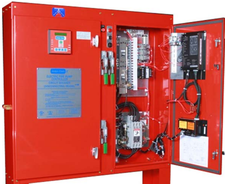
Transfer Switch Controller
